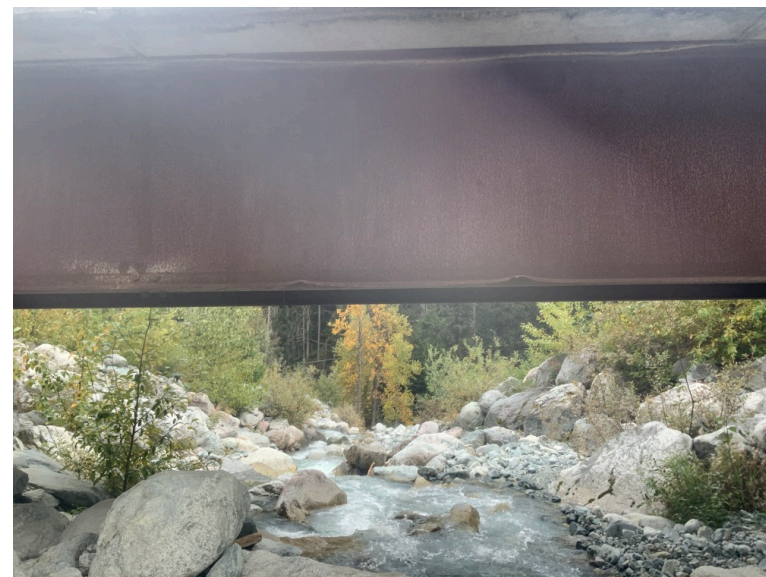
Superstructure, damage from debris
